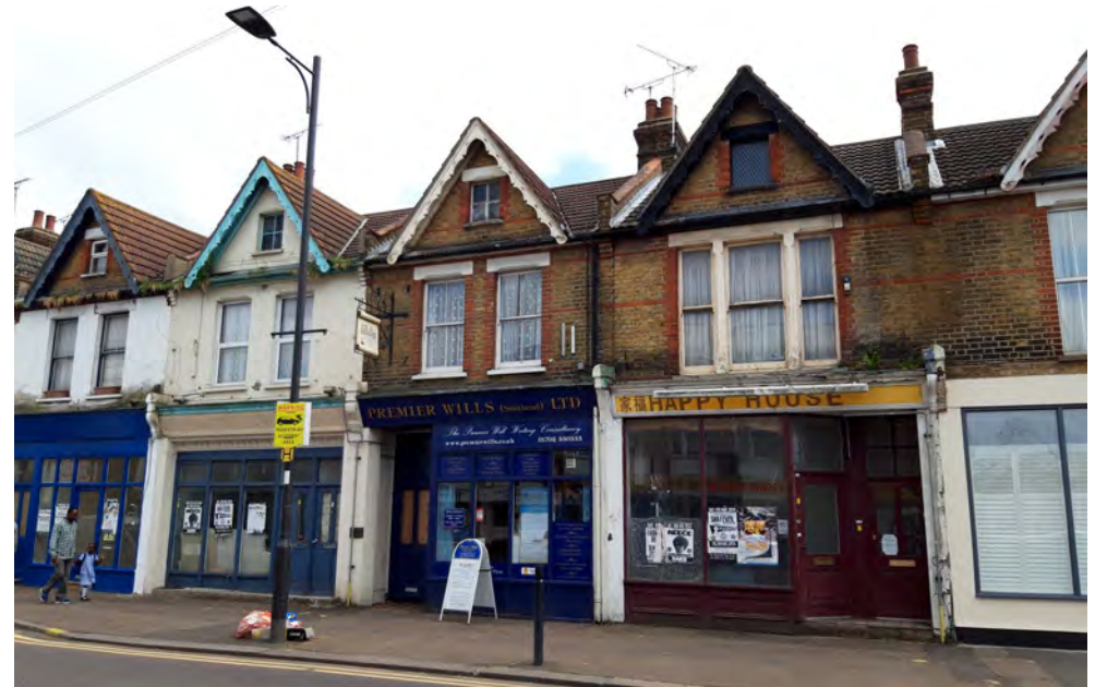
Issues with condition, such as poor decorative repair and problems with damp, indicated by vegetation growing out of blocked gutters.
