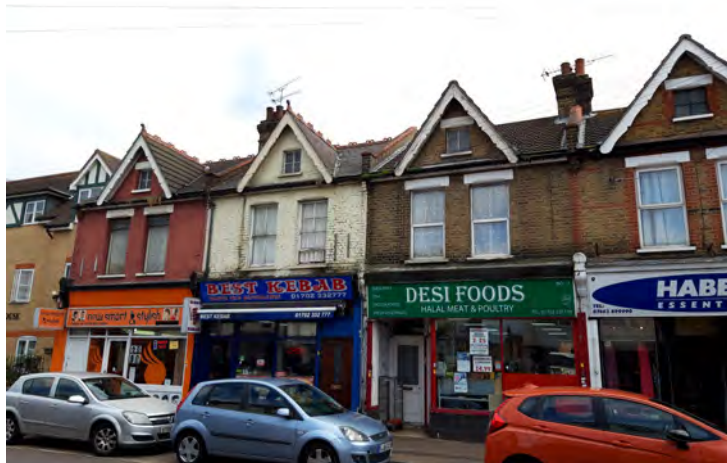
Oversized and garish shop fronts, plus painted brickwork and inappropriate replacement windows. The white painted building does have historic timber sash windows, though in poor decorative repair
