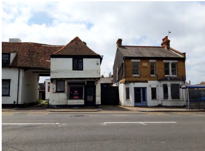
Two vacant buildings on Victoria Avenue where issues with condition are visible, including poor decorative repair and cracking to plasterwork
