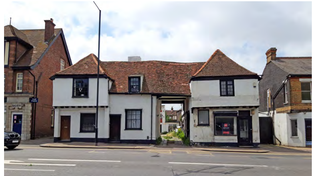
Nos.269–275 Victoria Avenue displaying jettied timber frame, gabled H-plan house and later windows and doors
